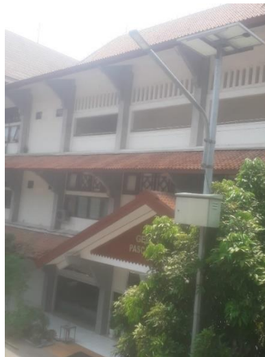
Gambar 3.9 Lampu Panel Surya di FEB UNS
